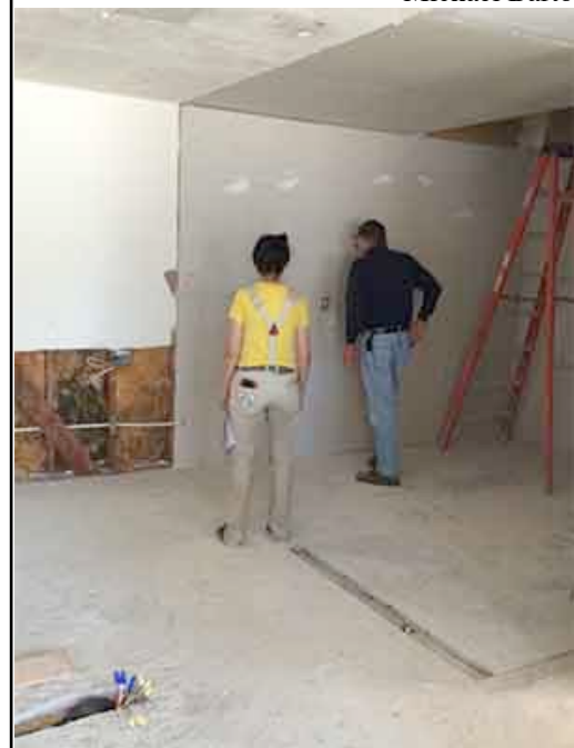
HB City Inspector checks work done on "Heartbroken" homeowner's condo.
